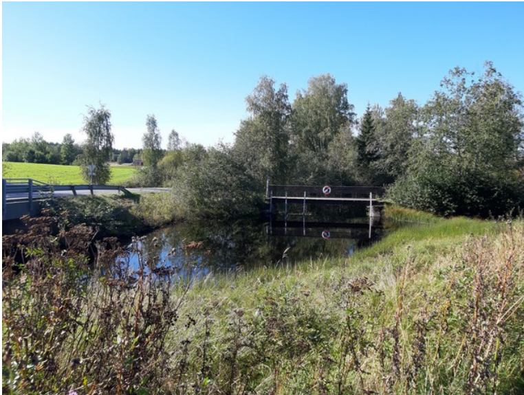
Here we have driven on to the Auli mill . Here we see the dam.
